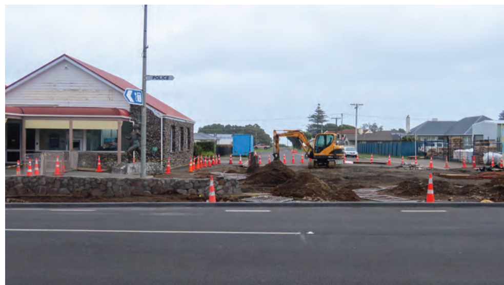
Concerns have been raised at the place which Ian Baker's wall will have as part of the Green Space development.
